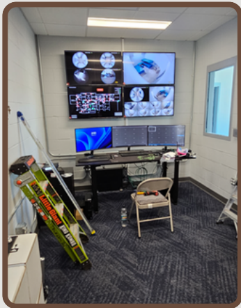
Tribal PD Control Room
