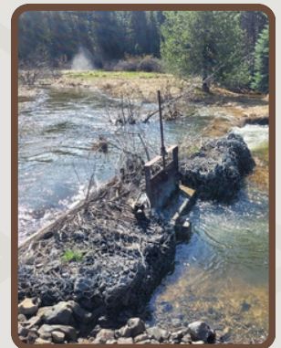
Musselshell Creek diversion that was failing
